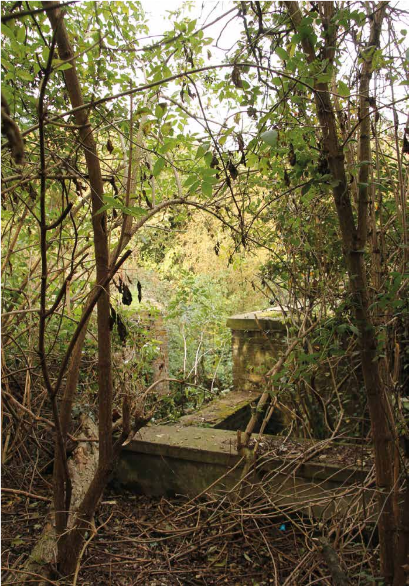
View 1: Part of the battery structure showing the undergrowth which has grown up around it.
